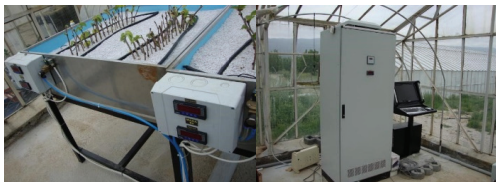
Figure 2. Computer-controlled system for temperature and humidity
