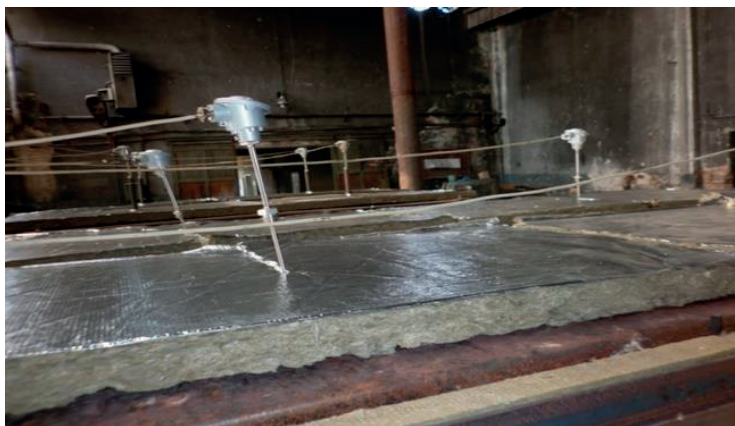
Figure 5. Temperature measurement system in the pyrolysis installation's reactor
