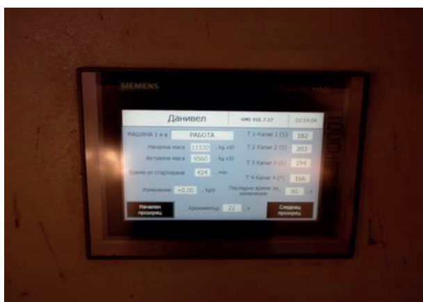
Figure 4. System for monitoring and setting of modes management of the pyrolysis installation
