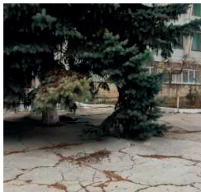
Figure 7. Degradation of asphalt path of ekranic Technosols by deformation cracks and perforation under influence of Picea sp. rooting
