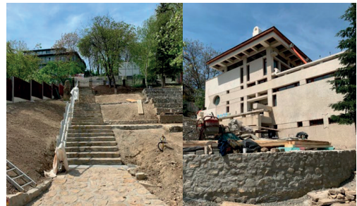
Figure 2. Existing situation (steps to the main access (left); amphitheater and "Bojdeuca Ion Creangă" Museum building (right))
